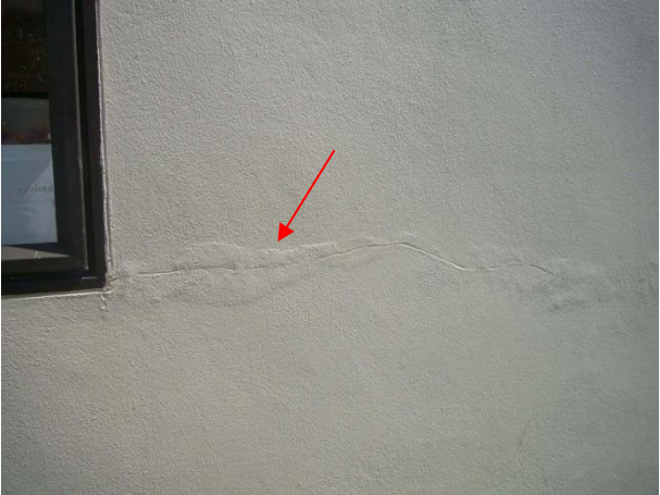
Cladding re-opening following a repair due to continued water ingress
