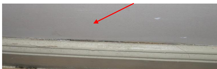
Cracked skirting board
